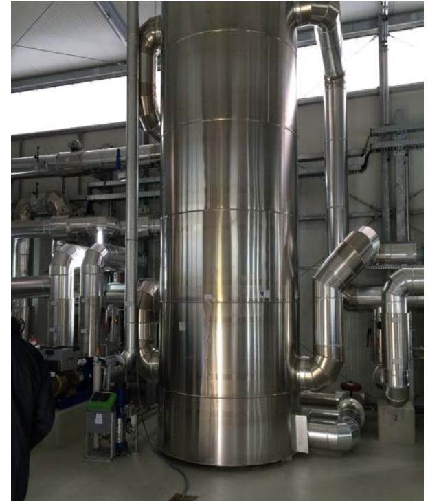
© Energiezentrale Senftenberg (ThEGA)
